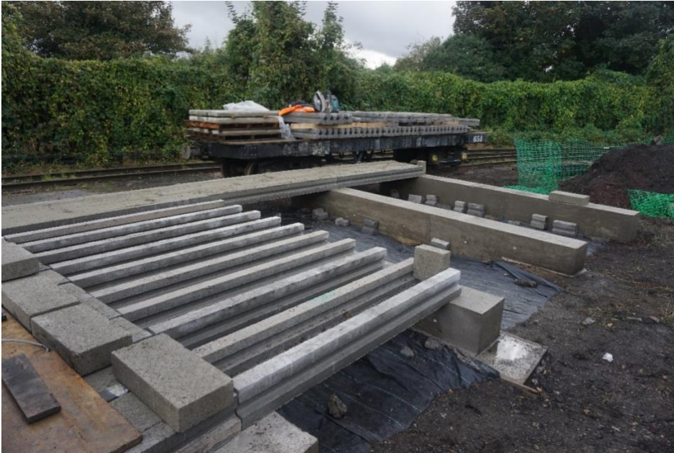
Image DSC05159.JPG. Sittingbourne Viaduct platform under construction showing the concrete beams being laid on the cast concrete piers ready for insertion of the concrete blocks and screed [P. Williams]
