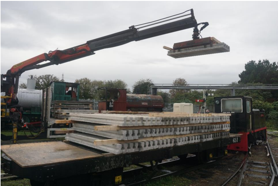
Image DSC05148.JPG. Butterley pulp wagon 651 behind ex-RNAD 4w DH Hunslet 6651 of 1965 Barton Hall being loaded with Ibstock concrete beams at Kemsley Down ready for transfer to Sittingbourne Viaduct [P. Williams]
